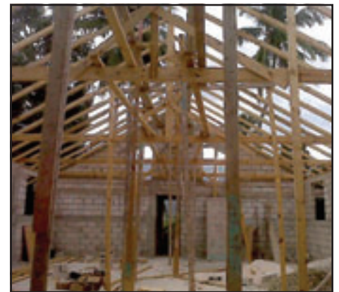
ABOVE: Much progress had been made on the church rafters by the last day. LEFT: Sunday was a day for church and rest.
