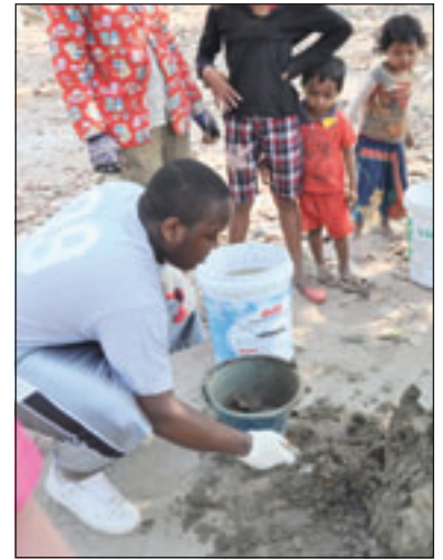
Christopher Blair, left, mixes cement that will be used to secure fence posts in the ground.
