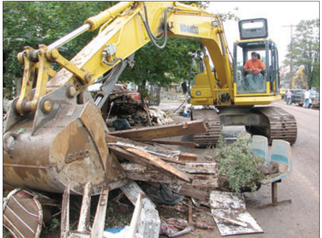
Heavy equipment filled the Main Street of Prattville, N.Y., as household goods destroyed by the flooding were hauled away.
