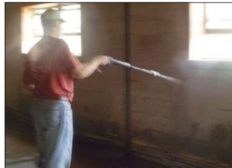
ABOVE: Rev. Dale Ashby power washes a basement. RIGHT: Rev. Wongee Joh, right, and her volunteers from Holmes UMC.
