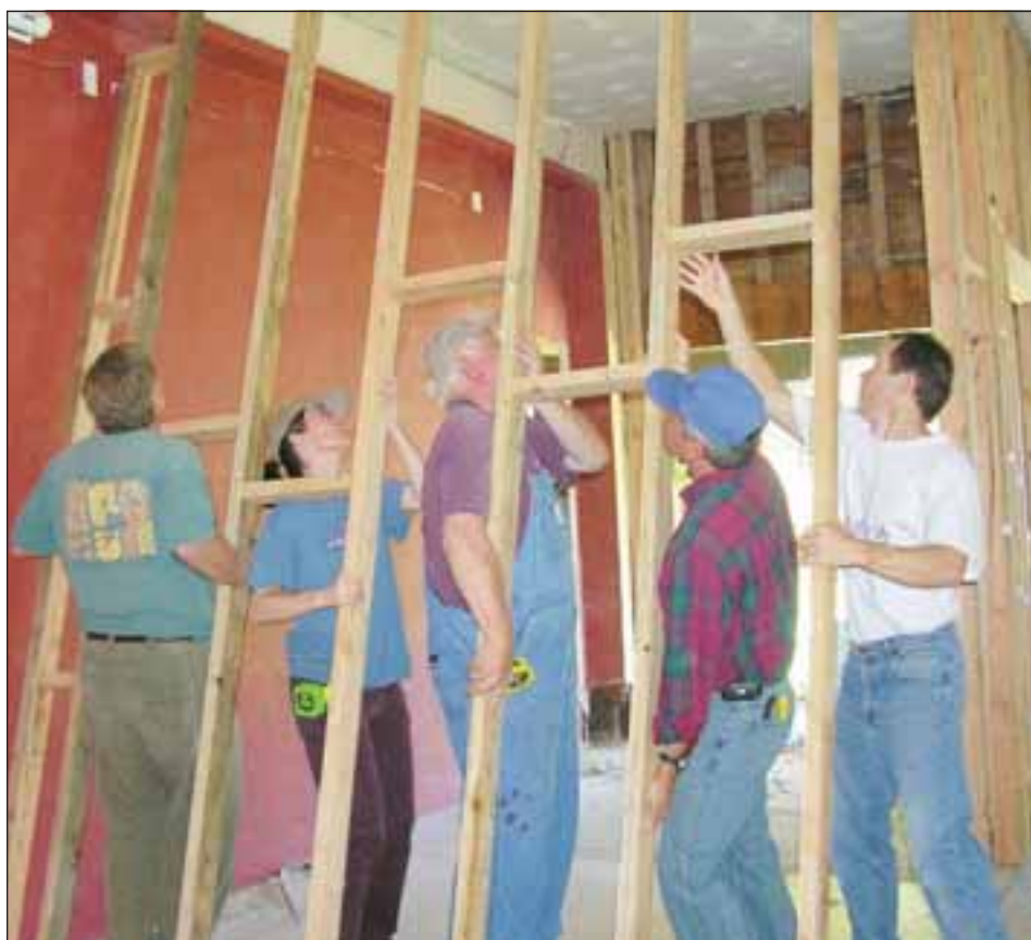
Bill Burnside, Shannon Cobb, George Woodring, Jose DaCruz and Mark Konopka raise a wall to create a new foyer in the carriage house.
