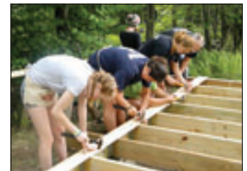
Participants in the Woodsmoke program work on the tent platform, above, and pour concrete for the platform footings, at left.
