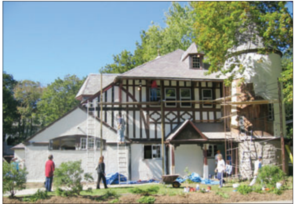
Exterior renovations on the carriage house in October 2008 were the first work project.
