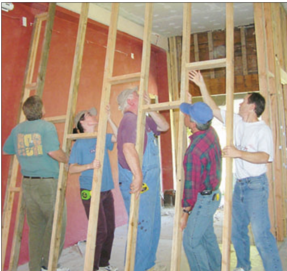
Bill Burnside, Shannon Cobb, George Woodring, Jose DaCruz and Mark Konopka raise a wall to create a new foyer in the carriage house.
