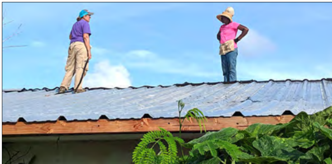
Linda Mellor, left, and Matilda Vandepuije atop a roof they were repairing in Saipan. Below, the team takes a break; from left are Carlos Figueroa, Art Mellor, Linda Mellor, Bob Snyder from Georgia, and Matilda Vandepuije.
