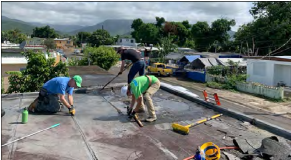
Above, rooftop work included preparation for waterproofing; below, members of the team take a photo break in the 90° heat in Puerto Rico.
