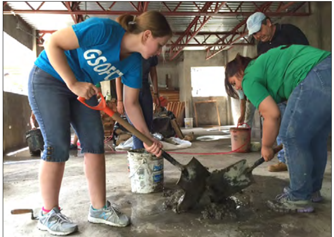
Mixing up concrete to trowel on the walls was not always an easy task.
