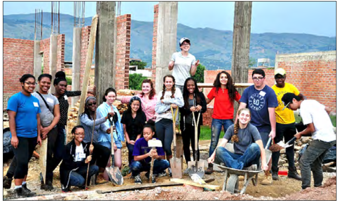
Youth Ambassadors in Mission stop for a team photo at the construction site; below, lunch brings smiles all around.
