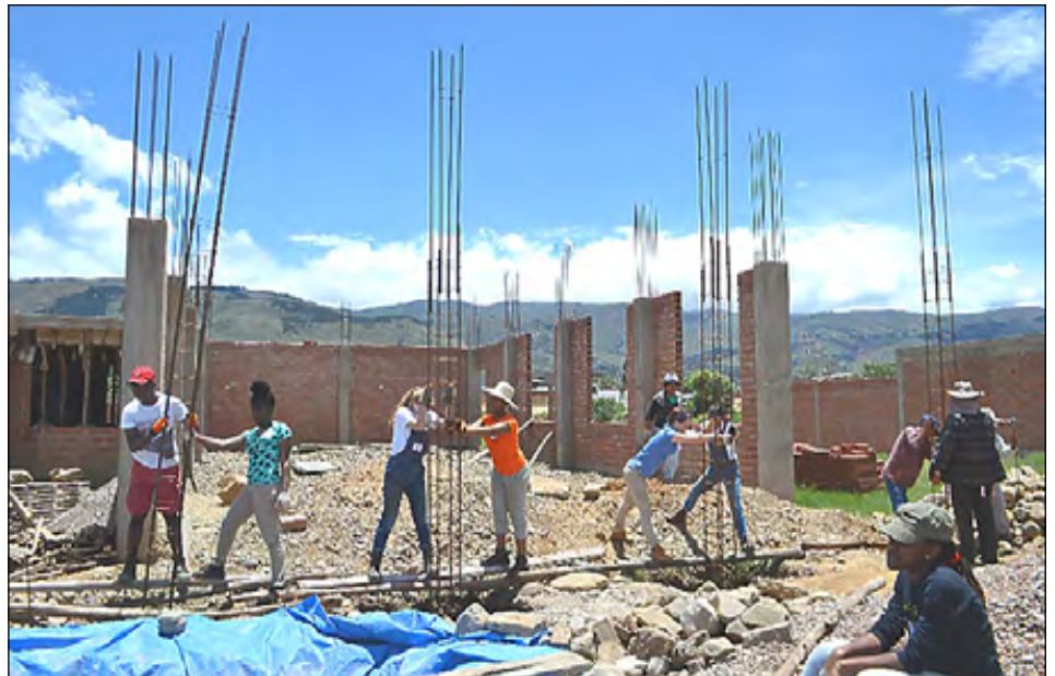
Youth work together to stabilize rebar as part of a construction project in Cochabamba, Bolivia. Below: Children delight in the gift of new crayons.
